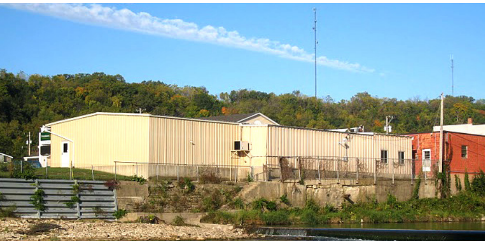
Collapsing river access steps and high floodwalls will be modified in the Spring of 2014 to better connect the community to the new river enhancements.
