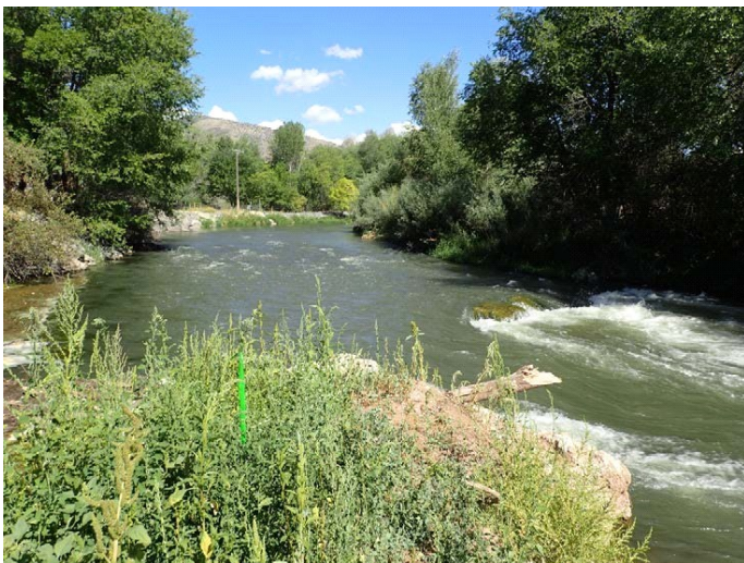
Pentz-Smith irrigation diversion structure before restoration. The grade control created either too large a head drop or high velocities that blocked upstream aquatic movement.
